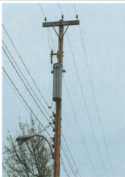
Brock St. Pole Transformer non-PCB
