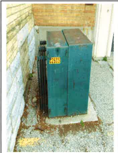
Transformer located on West side of the Main Building.
