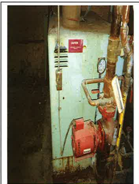
Former gas heater in the basement Utility Room
